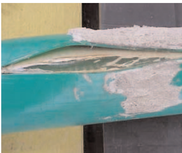
FIGURE 3. Split of secondary pipe; apparent failure of primary layer underneath
