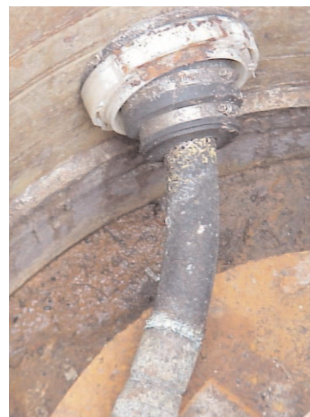
FIGURE 1. Black mold growth; degradation of single-walled pipe's external cover
