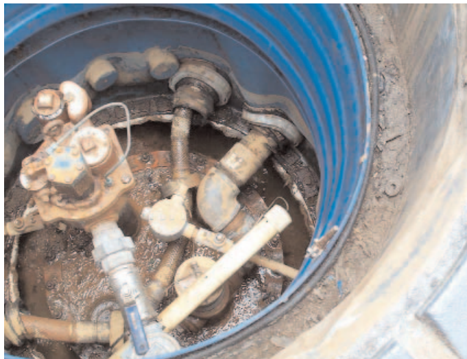
FIGURE 4. Ripple in sump wall; torn boots; shift in pipe position within secondary pipe
