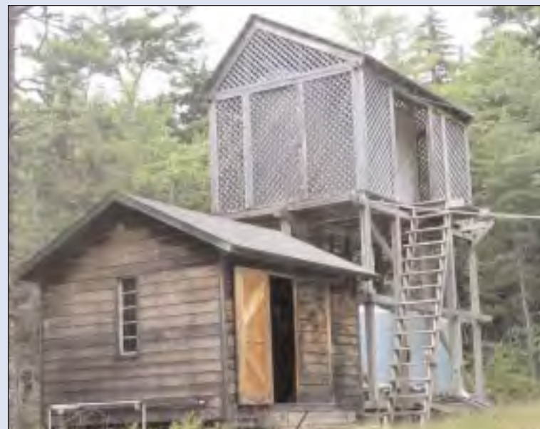
Small System, Big Success At the top of a hill on Maine's MacMahan Island sits the only (for now) drinking water desalination facility in New England. The building on the left houses the plant's two desalination units; the structure on the right contains the water holding tanks.
