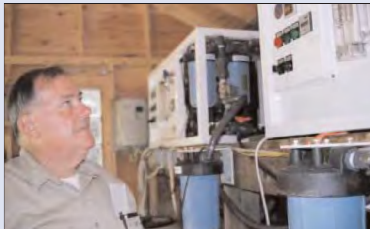
Eyeing the Investment MacMahan Island superintendent Peter Schuerch monitors the performance of a desalination unit as it converts seawater into fresh drinking water for the island's residents.
